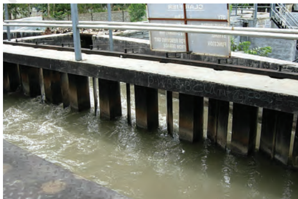
Fig. 13.4 Grit and sand removal tank
